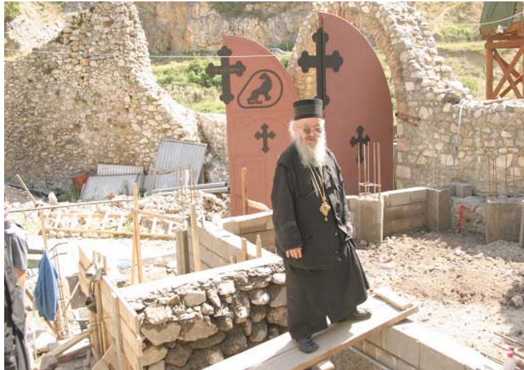
Vladika ArĀemije obilazi gradilište pri obnovi manastira SveĀih ArĀhangela His Grace Bishop Artemije visits the building site during the renovation of Monastery St. Archangels
